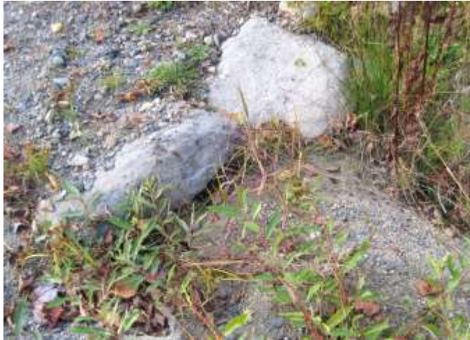
Blocked culvert in North Country Region
